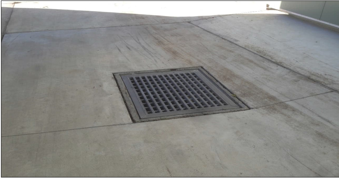
Figure 7-2: Directive Drainage – Elf Farm Site
