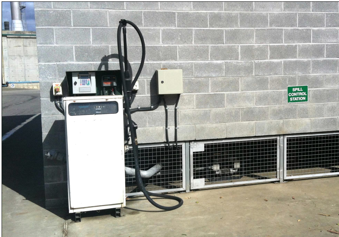
Figure 7-1: Spill Control Station and Signage – Elf Farm Site
